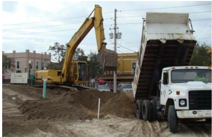
Eustis Public Works personnel begin site preparation for sod and pathways on the Foundation property.
